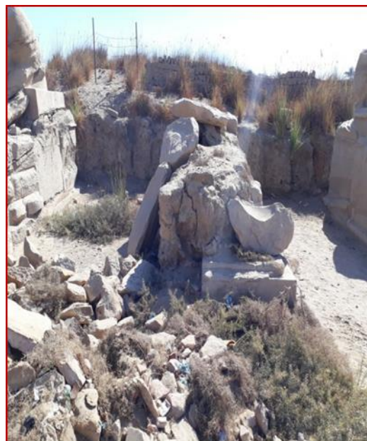
Fig (7). The condition of some of the bases of the road, which are destroyed and weeds spread, and the presence of cracks and many separations is noted
