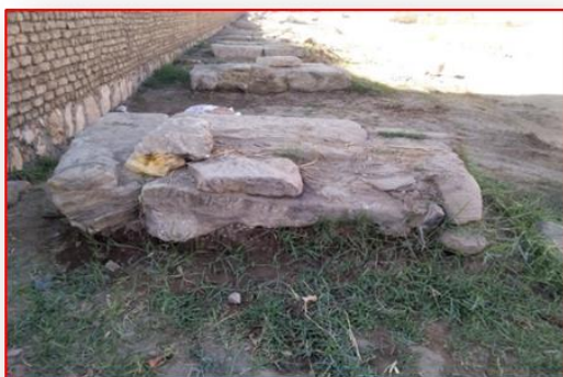
Fig (4). Shows the condition of some of the bases that were found and the effect of the various deterioration factors on them, only a course or two of its stones remain, and a great loss has occurred in them
