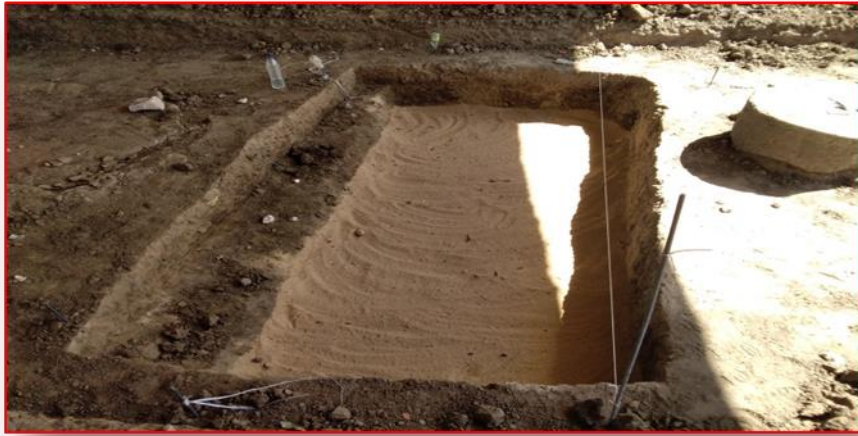
Fig (12). The shape, depth and dimensions of the hole on which the base is built and the replacement of sand and fine gravel is placed in it
